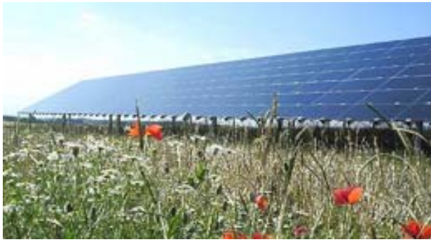
Figure 1: Thin-film CdTe 1,400-kW thin-film solar installation.
